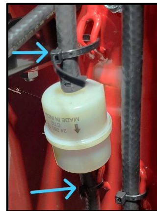
Figure 3 Zip Ties Securing Fuel Filter
