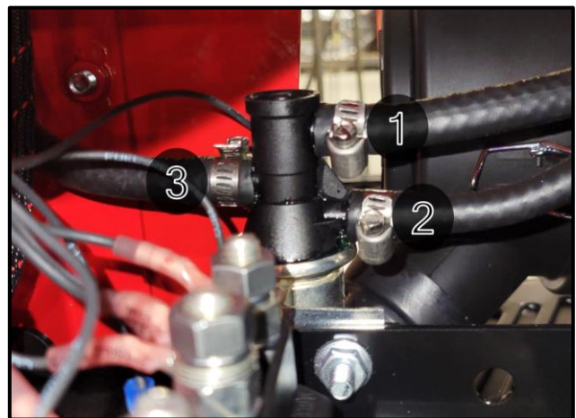
Figure 16 Labeled Fuel Transfer Switch
