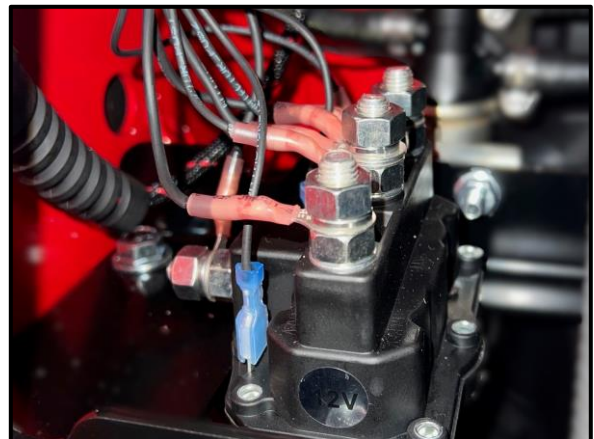
Figure 25 Contactor on Battery Tray
